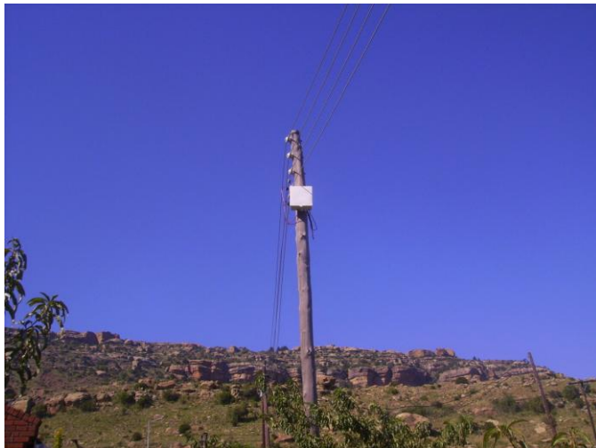
Figure 5: complete installation at Phuthaditjhaba
